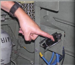
1 Power to the aircraft is switched on by means of the ground flight switch, aft of the forward main spar
