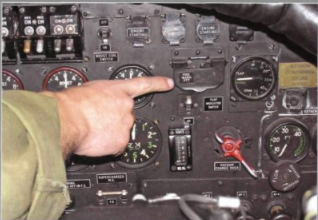
6 The fire system light test is carried out to ensure that the system is working
